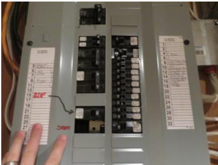
Figure 12 Open Slot(s) at Main Service Panel
