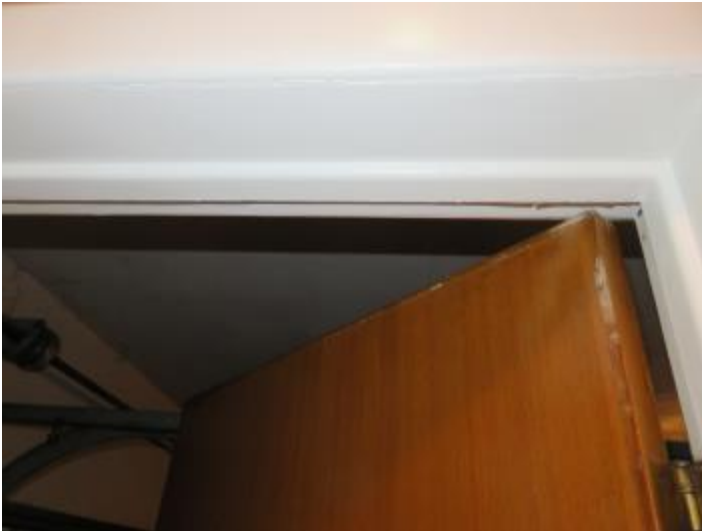
Figure 22 Entry Door not Fire-Resistant/Missing Closer
