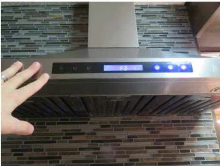
Figure 19 Range Hood Fan(s) Noisy/Vibrating
