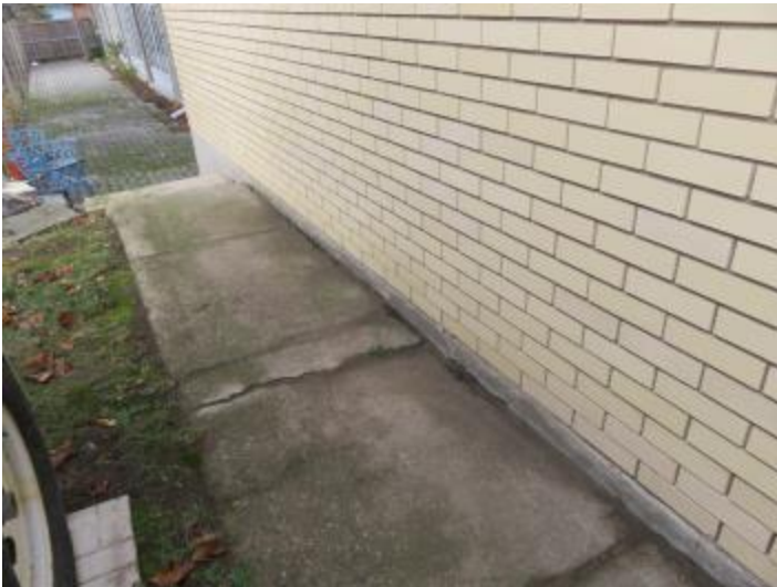
Figure 1 SW Walkway Minor Deterioration
