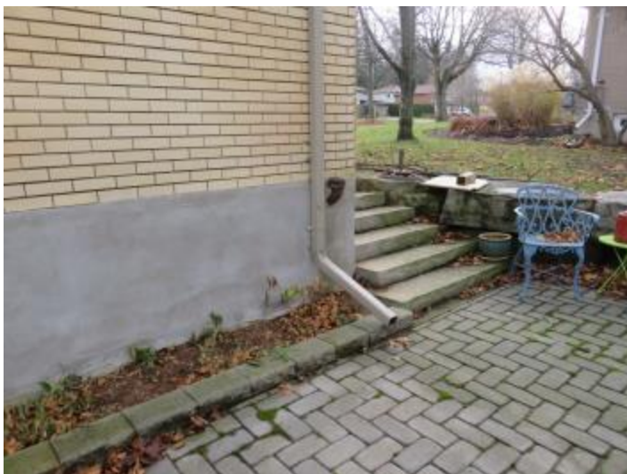
Figure 7 NW Downspout Discharges onto Walkway
