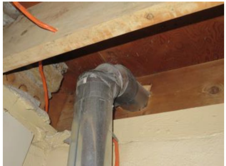
Figure 18 Duct Tape at Dryer Vent Joint(s)
