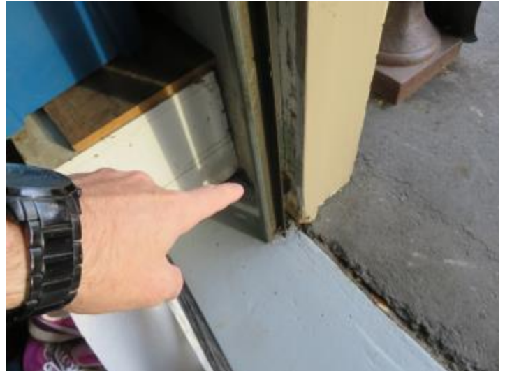
Figure 23 Vehicle Door(s) Missing Sensor(s)
