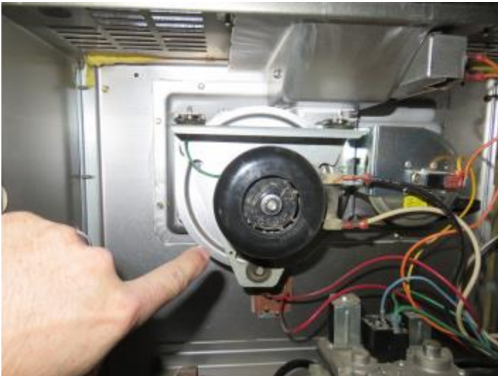
Figure 13 Furnace Inducer Fan Noisy
