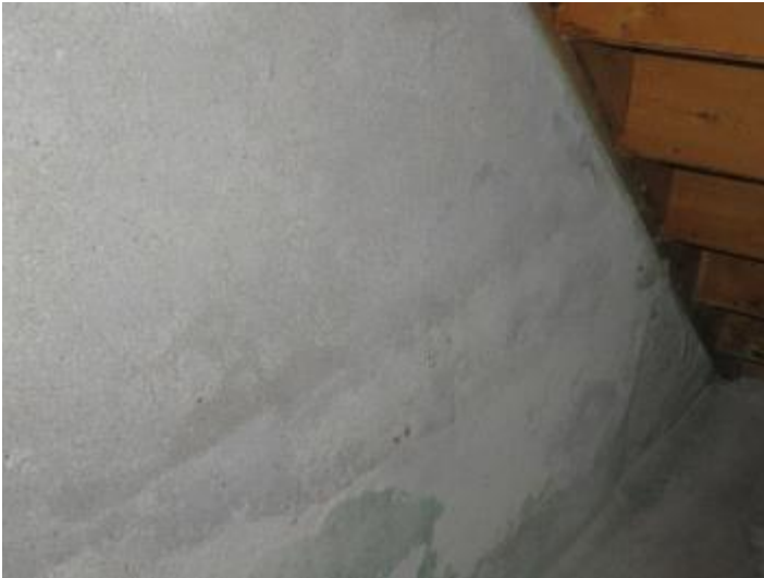
Figure 10 Evidence of Moisture SW Wall(s)
