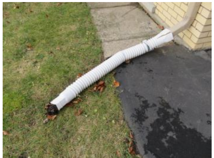
Figure 8 Debris in SW Downspout
