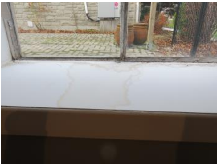
Figure 20 Staining at NE Basement Window
