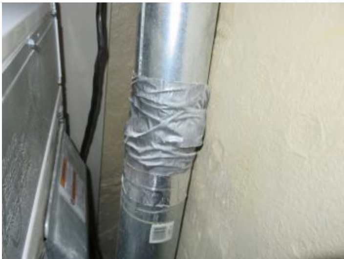
Figure 17 Duct Tape at Dryer Vent Joint(s)
