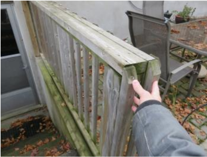
Figure 3 Back Stairway Loose Guard(s)
