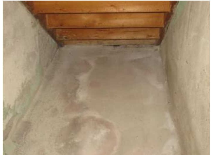
Figure 11 Evidence of Moisture SW Wall(s)
