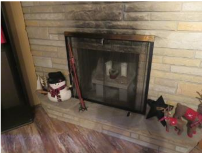
Figure 15 Recommend Specialist Evaluate Fireplace
