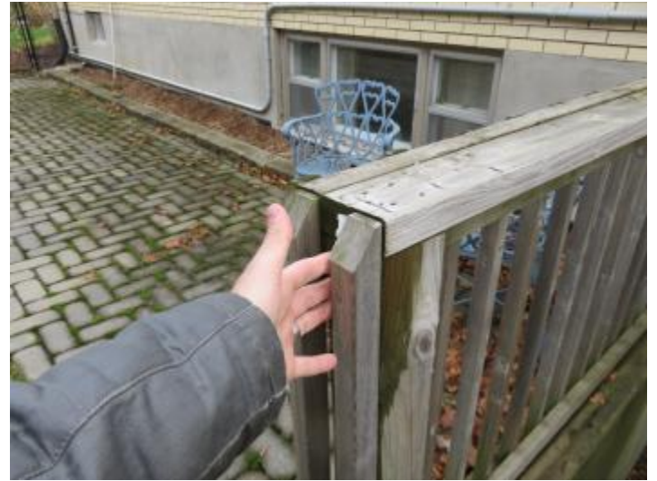
Figure 4 Back Stairway Loose Guard(s)
