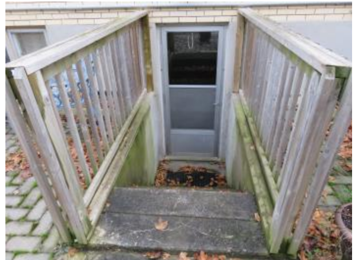
Figure 2 Back Stairway Missing Handrail(s)
